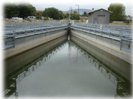
Figure 2 - A Canal Fish Screen
