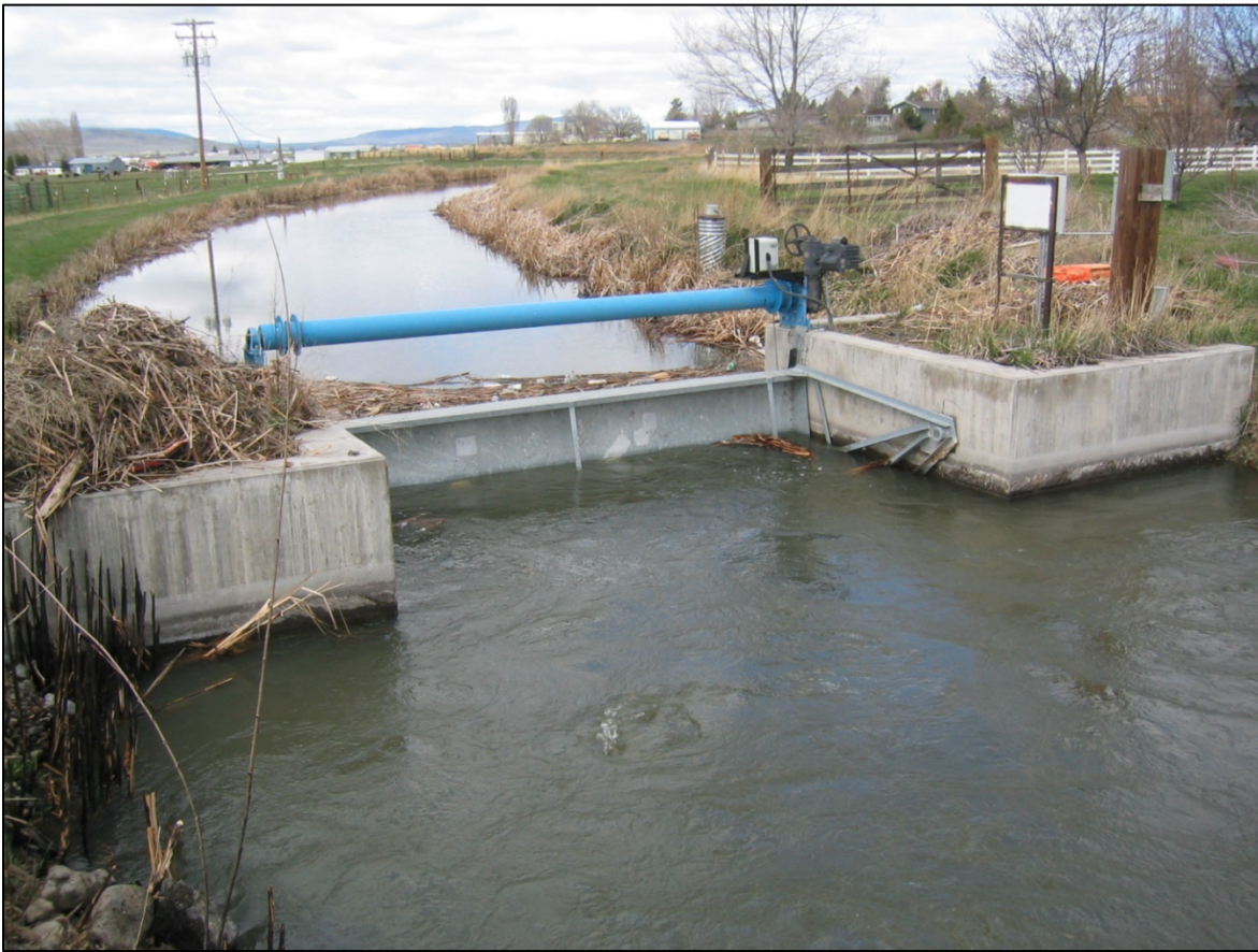
Figure 64 B Canal Automated Gate – Attempts to fully Automate this Gate since 2011 have failed.
