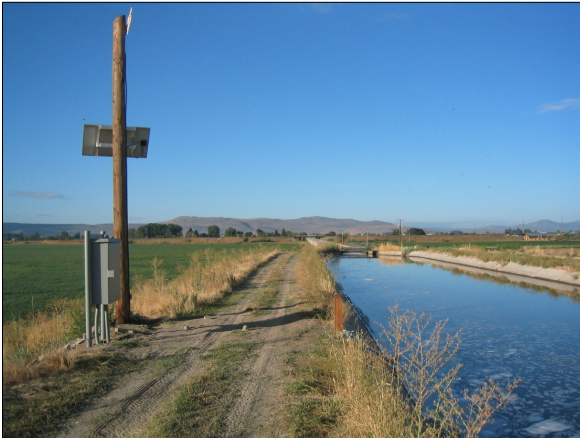
Figure 66 Upper C Canal SonTek Measurement Station
