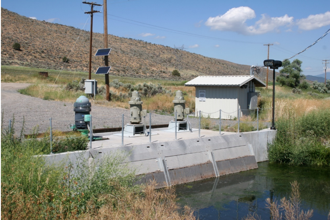
Figure 69 Miller Hill Pumping Station
