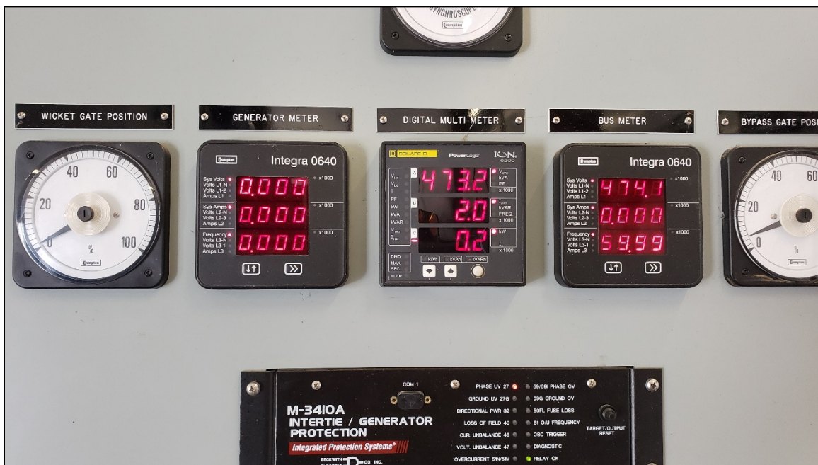
Figure 62 C-Drop-Hydro Power Measurements provided through C-D-H PLC Developed by Sorenson Engineering
