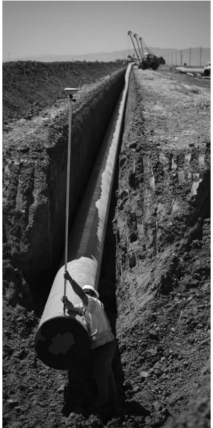
Installing irrigation pipe in California's Central Valley. Photo courtesy of Provost & Pritchard Engineering Group.
