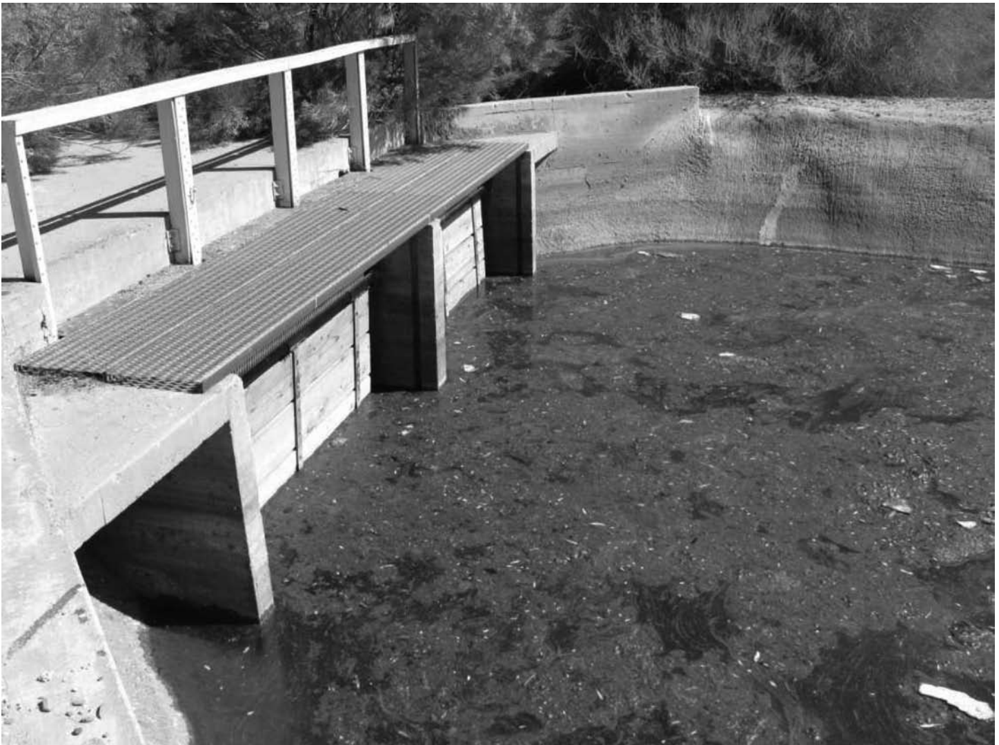
Weed and algae choked canal in Arizona. Photo courtesy of PK Gills
